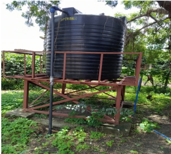
Plate 1: Piped Water storage tank in the compound in Malakal Teaching Hospital.
