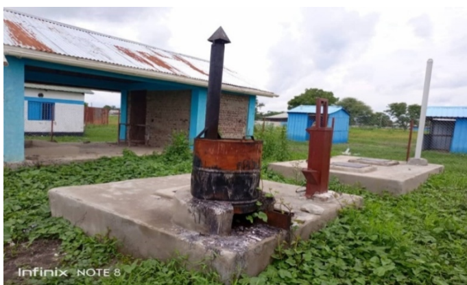
Plate 6. 2: Unprotected incinerator site in Asosa PHCC. Source: Author, (2025).
